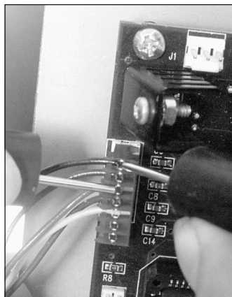
Testing for voltage at the red and black output wires on the back of the Sentry.
