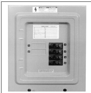
Know the location of the circuit breaker panel. Label the breaker that controls your kiln's circuit.
