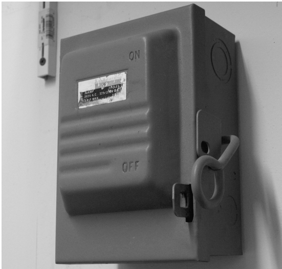
Large studio kilns should have a power disconnect box for the kiln. Place the box in the kiln room.
