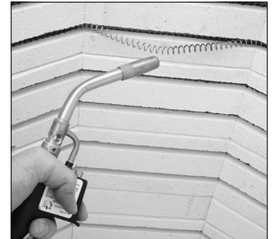
Using a propane torch with push button igniter to heat a bulging element.
