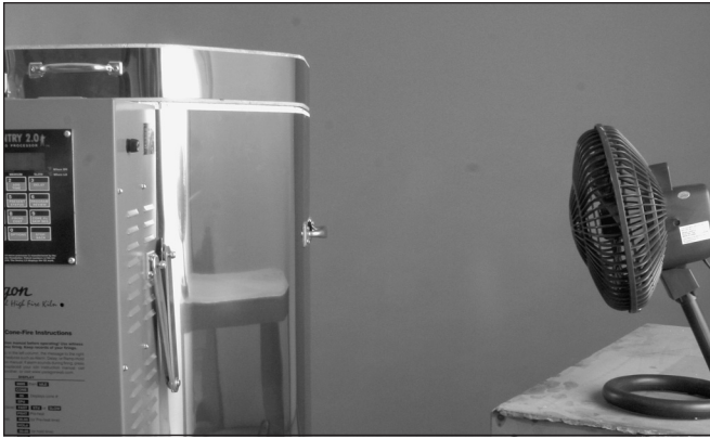
Lower the switch box temperature with air movement. This is especially useful during hot summers.
