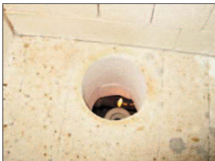
View of pilot from inside kiln.
