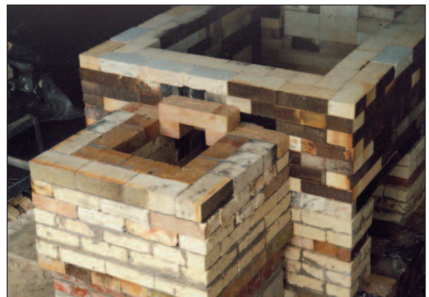
The first eight courses of the kiln and the first five courses of the chimney/collection flue in place, with a hard brick lintel spanning the flue/chimney opening.
