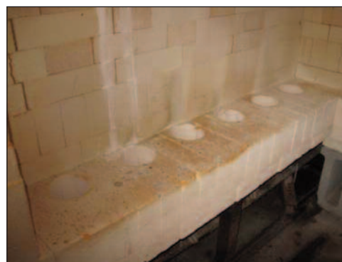
The burner ports.
