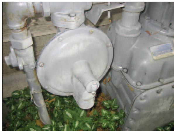
This natural gas regulator takes the gas coming into the house and reduces the pressure of it for use by household appliances.
